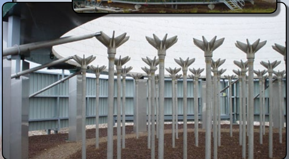
Enclosed Ground Flare with Interior Chamber Cast Burner Heads
